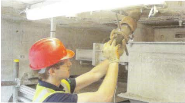
Figure 3. Cardox operative inserts and locks the specially designed silo tube into an Angled Socket.
